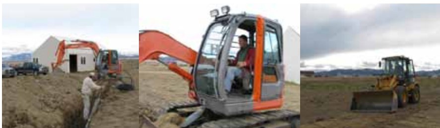
Steve Pelcher (l), Derek Brown (m) and Darrell Miller (r) work on getting water to the barn. Electricity is next!
